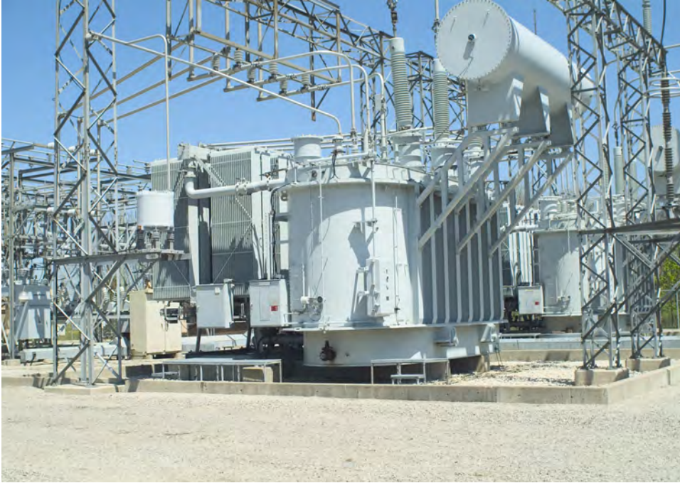
Three-phase transformer bank used for power distribution.
